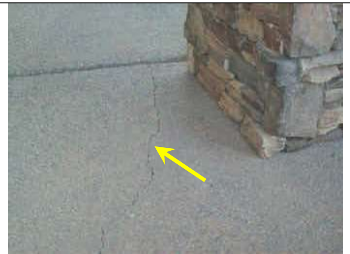
Photo 36: Distress crack on rear patio concrete slab.
