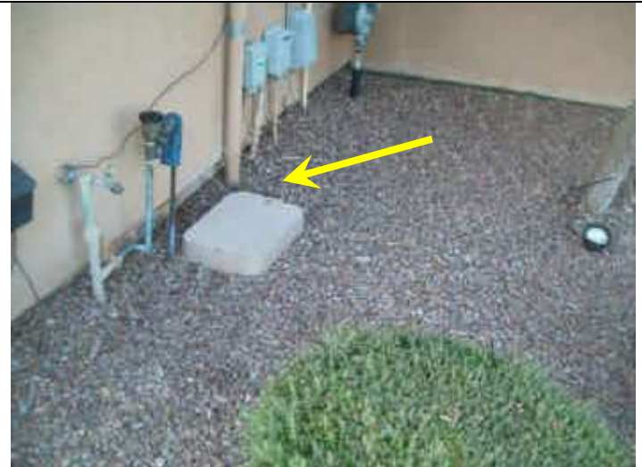
Photo 24: Front exterior view east end. Low spot and negative grade at utility entrances.
