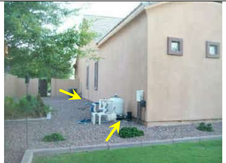
Photo 26: Rear exterior view east end. Low spot and negative grade. Signs of previous pool pump repair north end.
