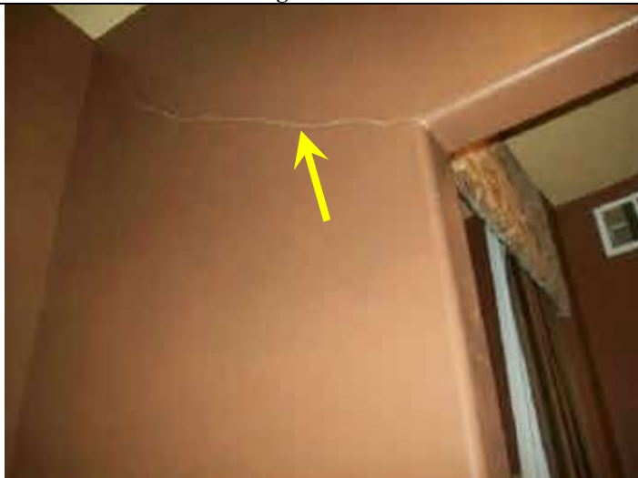
Photo 11: Hairline cracks on drywall at corner of interior door of guest room.
