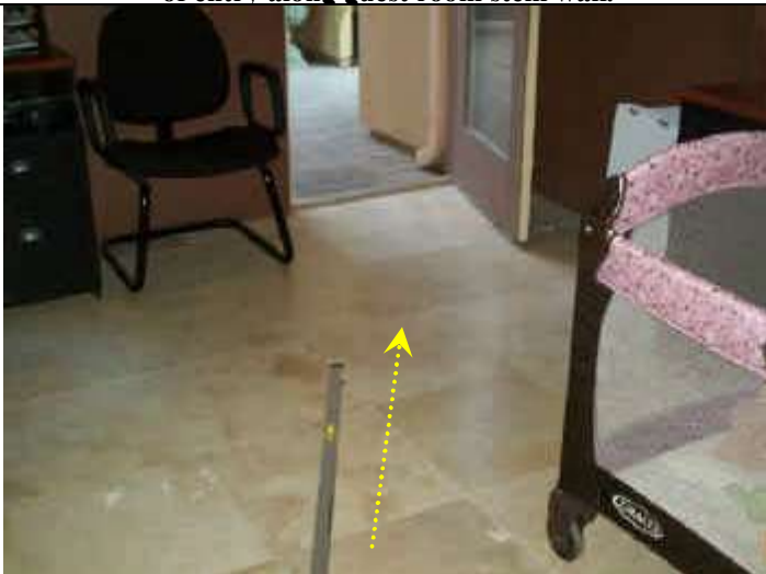
Photo 5: View looking east from guest room. Distress crack on floor tiles running diagonally through room.
