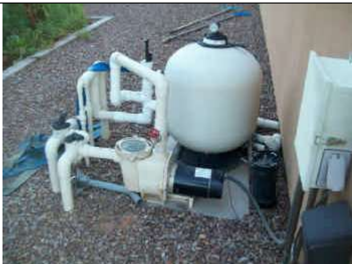
Photo 29: Rear exterior view east end. Signs of previous pool pump repair north end.
