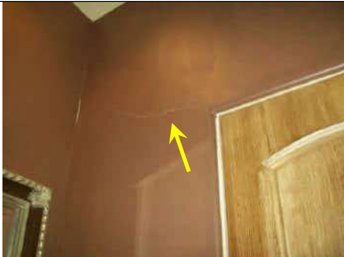
Photo 9: Hairline cracks on drywall at corner of entry door of guest room.
