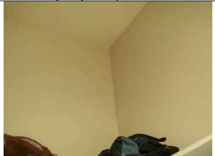
Photo 16: Distress crack in drywall of MBR closet area.
