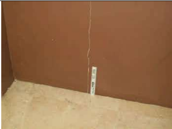
Photo 7: Hairline cracks on drywall of south wall of guest room.
