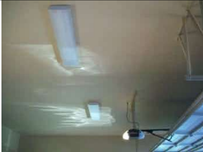
Photo 19: Distress crack on garage ceiling drywall.
