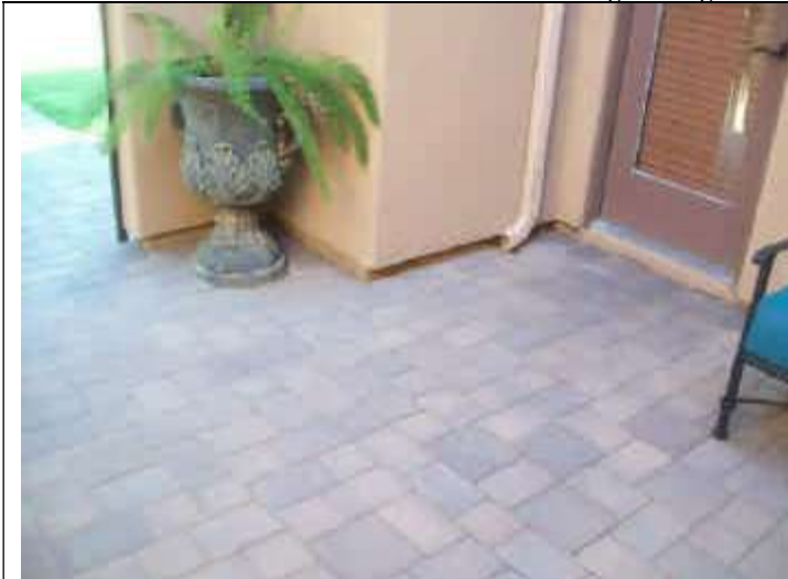
Photo 1: Front porch downspouts drain to west end porch and along guest room stem wall areas.
