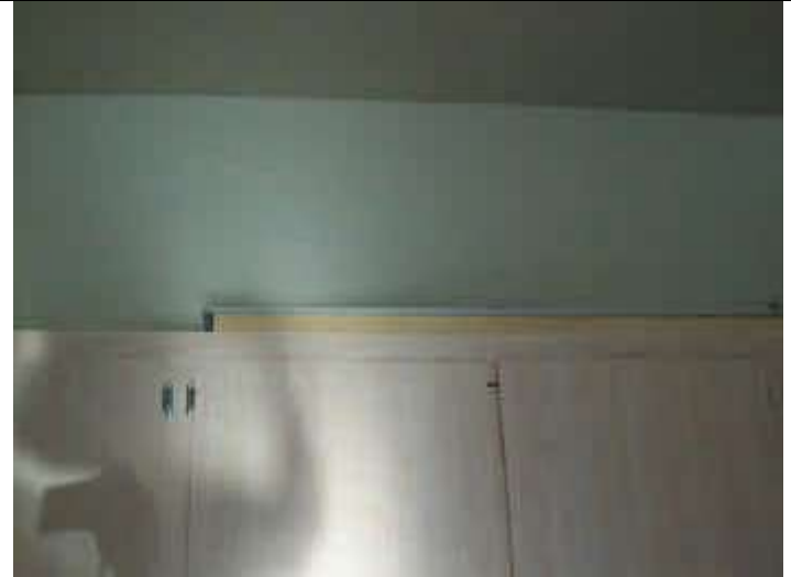
Photo 20: Distress crack on garage wall drywall above cabinets. .
