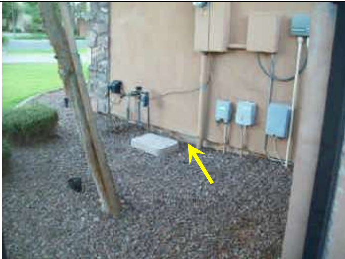
Photo 25: Front exterior view east end. Low spot and negative grade at utility entrances.
