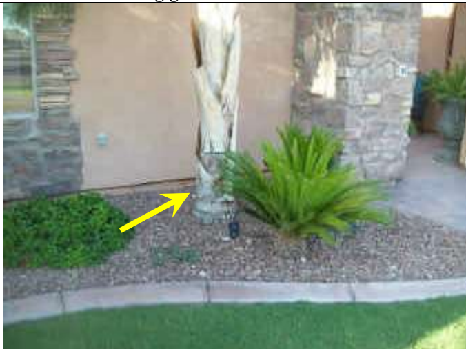
Photo 3: Low spot and negative grade front exterior just west of entry along guest room stem wall.
