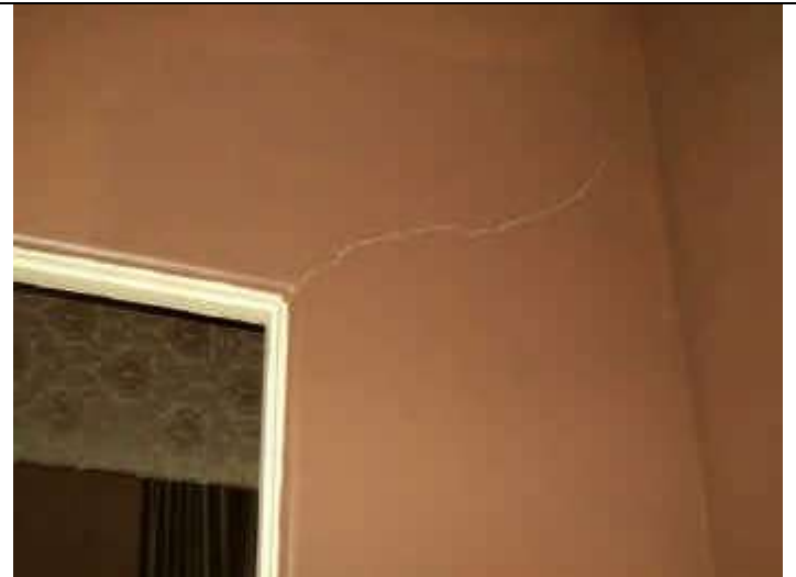
Photo 8: Hairline cracks on drywall at corner of interior door of guest room.
