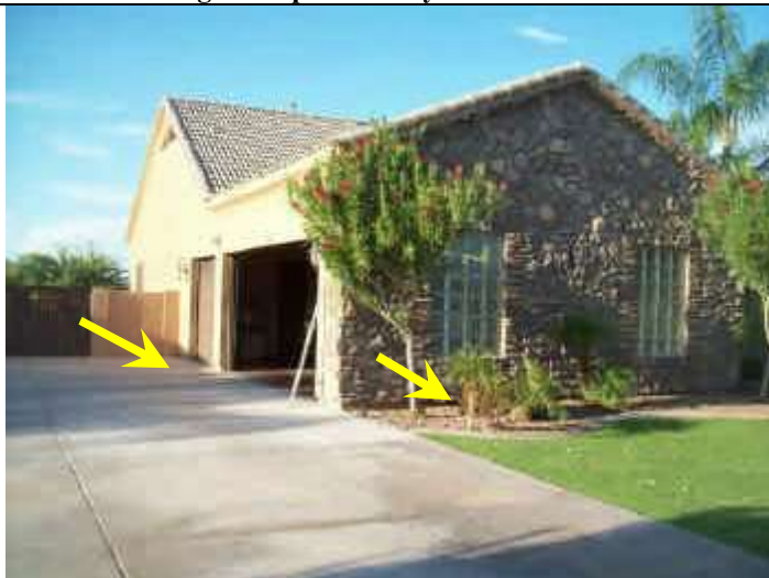
Photo 17: Front exterior view west end of home. Negative grade along garage south and west ends.
