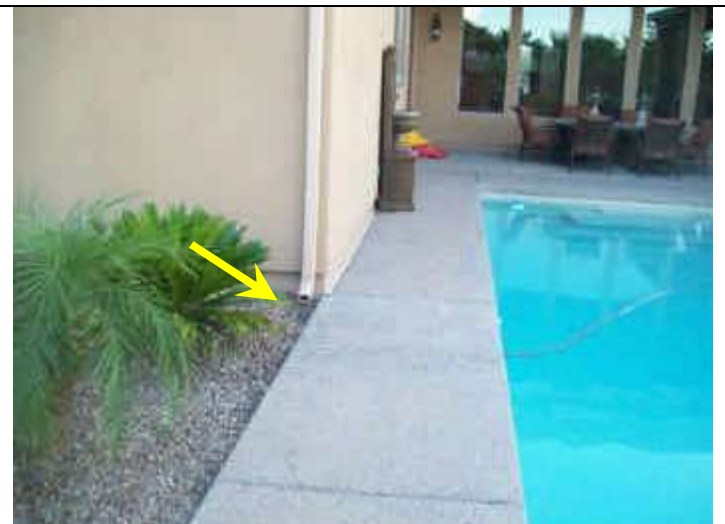
Photo 30: Downspout drains to rear exterior stem wall.
