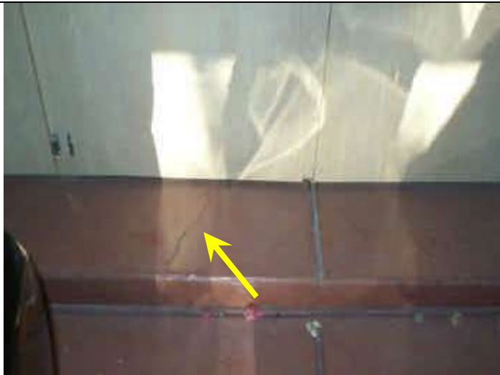
Photo 21: Distress crack on garage concrete at step up along east edge.
