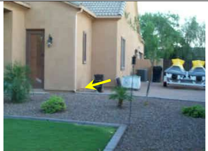
Photo 34: Rear exterior view west end. Downspout drains to stem wall.
