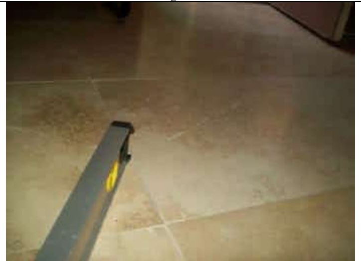
Photo 10: View looking east from guest room. Distress crack on floor tiles running diagonally through room.
