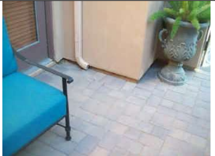
Photo 2: Front porch downspouts drain to east end porch and along main home stem wall areas.
