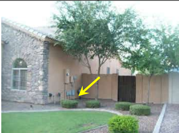
Photo 23: Front exterior view east end. Low spot and negative grade at utility entrances.
