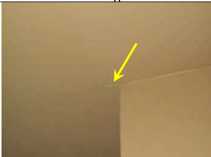
Photo 35: Distress crack on rear patio ceiling drywall.
