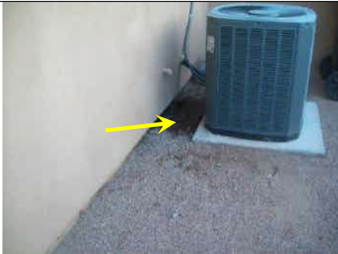
Photo 37: AC condensation line drains to stem wall along west exterior.
