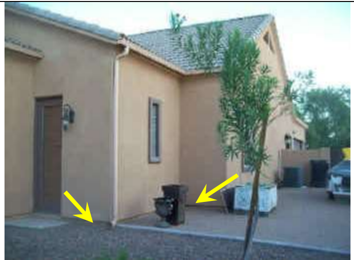
Photo 38: West exterior view. Downspout drains to stem wall and low spots noted along stem wall.
