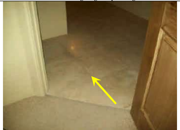
Photo 12: View looking down hallway in main home. Distress crack on floor tiles at entry to bedroom.
