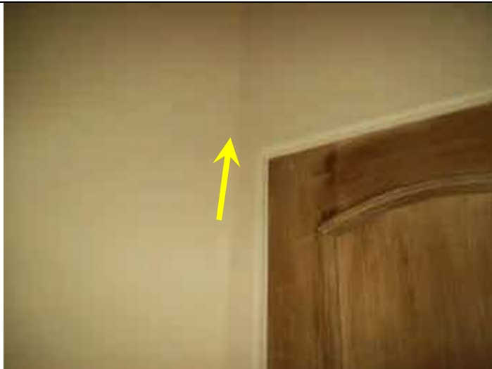
Photo 13: Hairline cracks on drywall at corner of interior door of bedroom.
