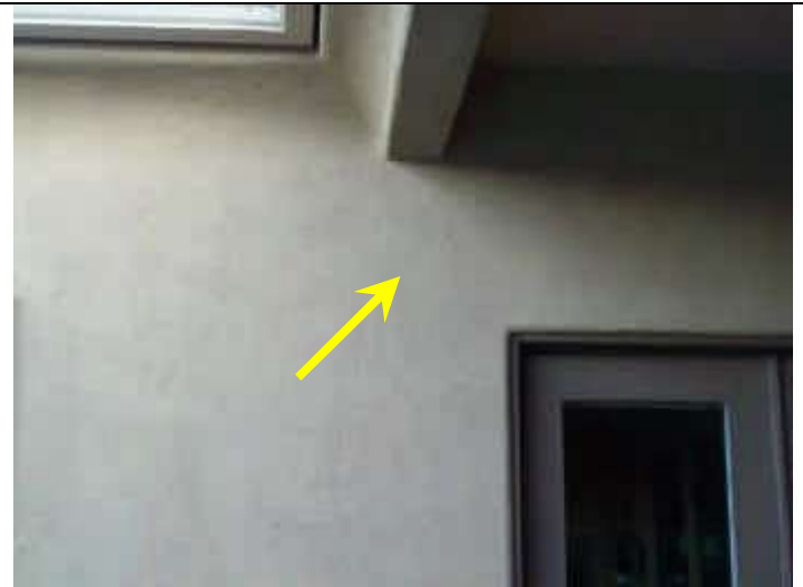
Photo 32: Distress crack on rear exterior stucco surface.
