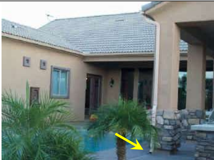
Photo 33: Rear exterior view. Downspout drains to patio column support.
