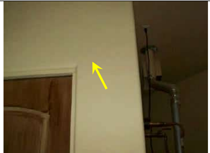
Photo 22: Distress crack on garage wall drywall above entry door. .
