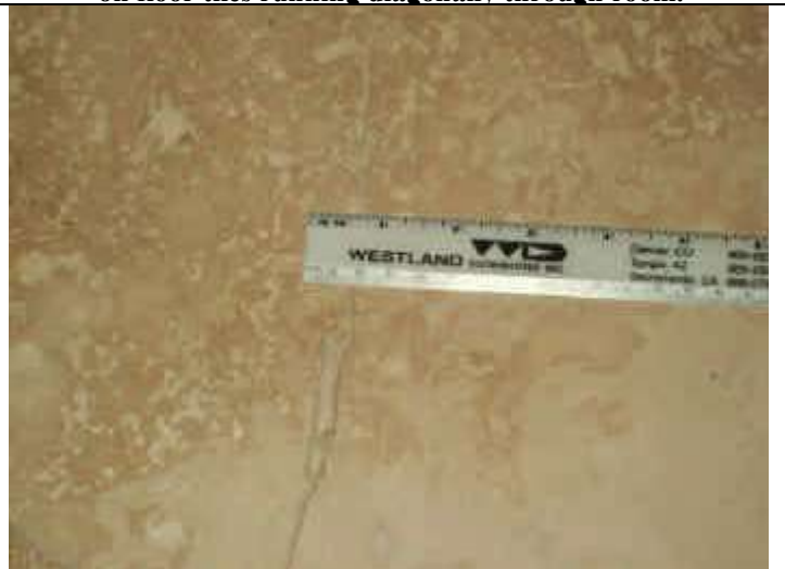
Photo 6: Cracks measured at less than 1/16 th inch in width with no vertical displacement in guest room.
